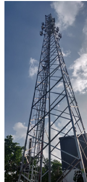
Bangalore - Roof Top Tower Tippenahalli
