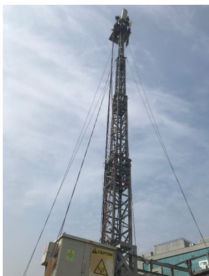
Mumbai - Cell on Wheels Bandra Kurla Complex
