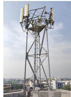
Delhi - Roof Top Tower Ajsar Management Pvt Ltd, Okhla Phase II
