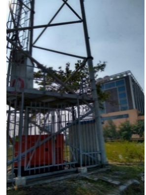
Kolkata - Ground Based Mast Rajarhat
