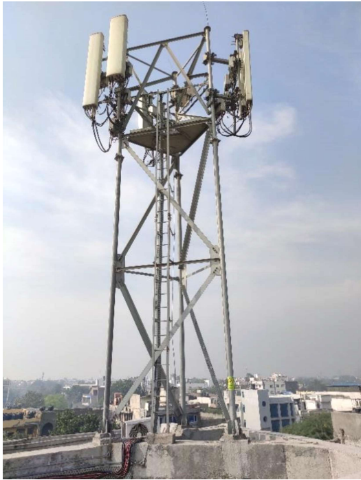
Delhi - Roof Top Tower Ajisar Management Pvt Ltd, Okhla Phase II
