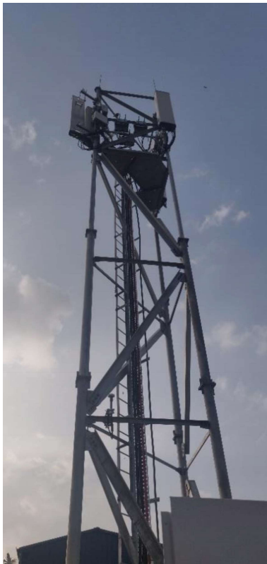
Bangalore - Roof Top Tower Rajaji Nagar
