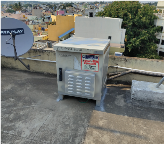
Sheshadripuram Kumara Park, Bengaluru
